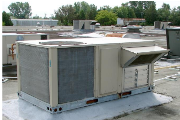
Figure 6-7: Example of a Rooftop Air Handling Unit
