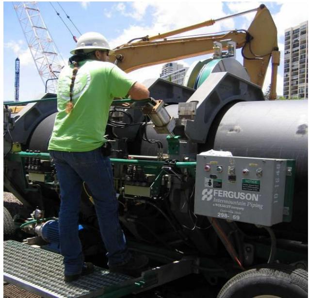
Figure 4-2: HDPE fusion used to join two lengths of pipe during the assembly process.
